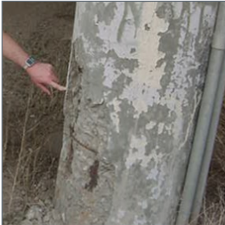
Damaged bridge column
