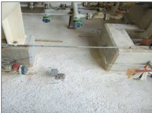
Concrete damaged by chemical attack
