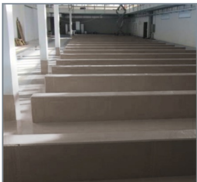
Unprotected storage area
